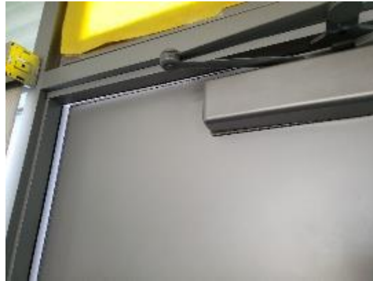
Figure 2. The spring-loaded door does not close by itself in classroom 207. When HVAC runs, it will lead to air leaking out of the space where the temperature should be adjusted.
