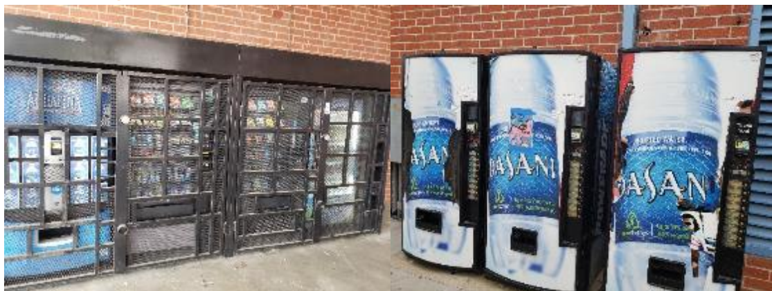
Figure 22. 8 caged vending machines near the cafeteria that could be equipped with a motion sensor vending miser. Also, six uncaged vending machines near the pool area by the bungalows.
