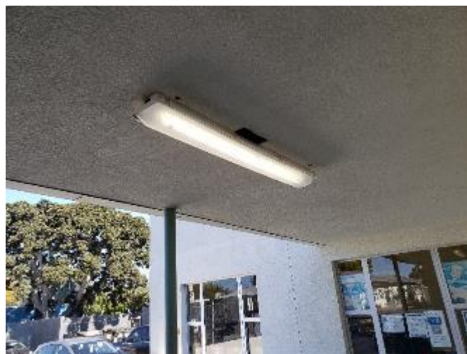
Figure 4. Exterior lights are on during the day near the cafeteria. It is recommended to have the exterior lights off during the day time.
