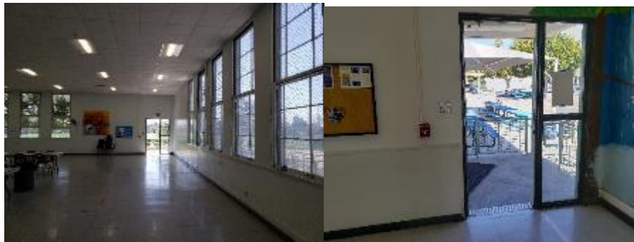
Figure 3. Exterior doors were wide open while the air conditioning is running in the cafeteria. It is recommended to have the doors closed while the unit is running.
