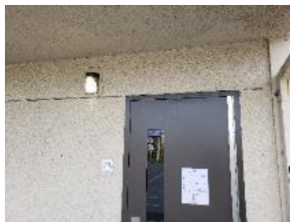
Figure 15. Exterior light was on outside of room B11.
