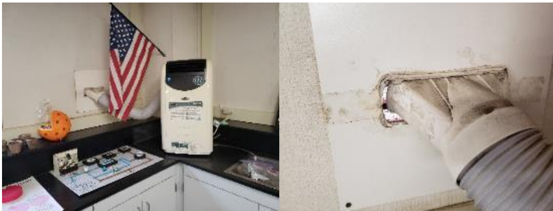
Figure 24. The air conditioning unit is not sealed well to the outside. It is recommended to ensure proper weather sealing during installation.
