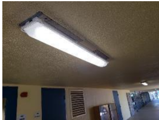
Figure 6. Exterior hallway lights on near the nurse's office during the daytime.
