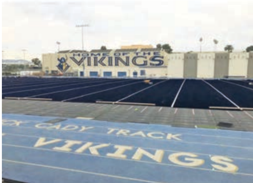
The new, blue turf, seen partially without its markings, will appear to be a lighter shade when fully completed with its cork infill.
