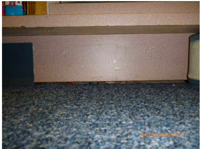
Photo #22: Overview of teachers cabinet toe-kick along north perimeter adjacent carpet staining
