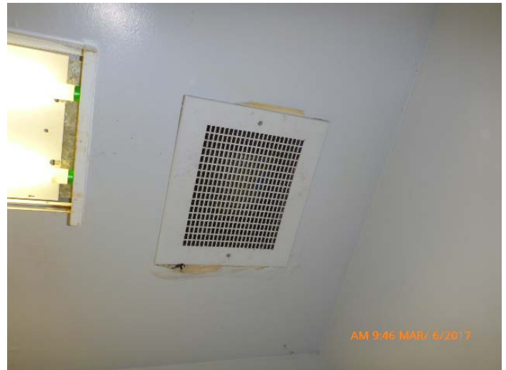
Photo 62: Moisture impact (e.g. damage) observed to ceiling in bathroom
