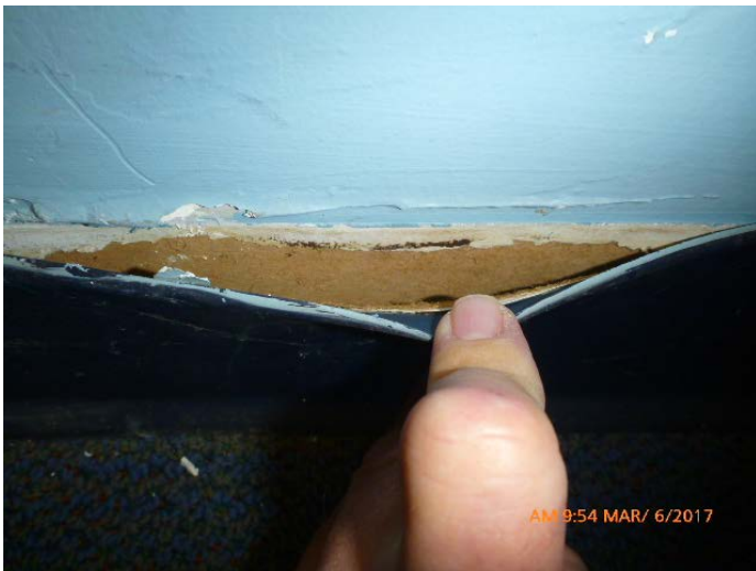
Photo 47: Mold growth observed behind base-cove on south wall
