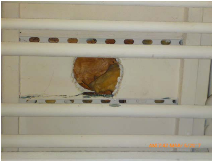
Photo #21: Hole observed in ceiling above stained carpet
