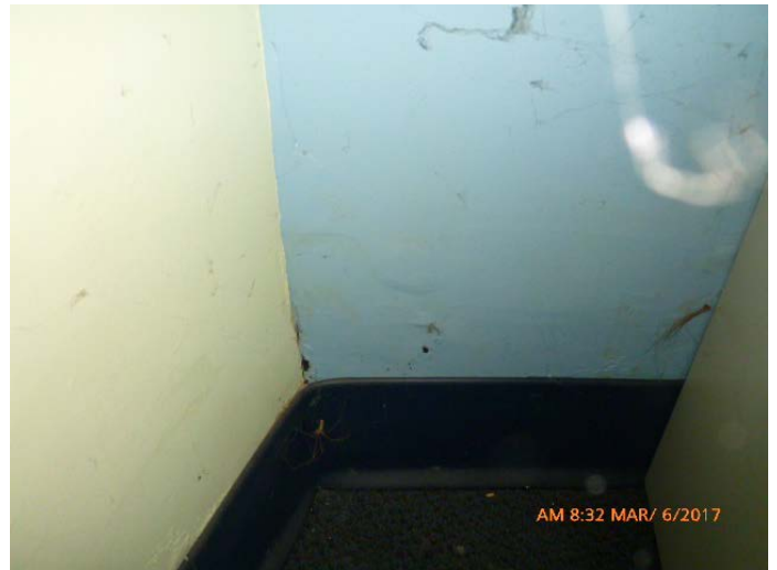
Photo #30: Overview of moisture damage along base of walls in NW corner
