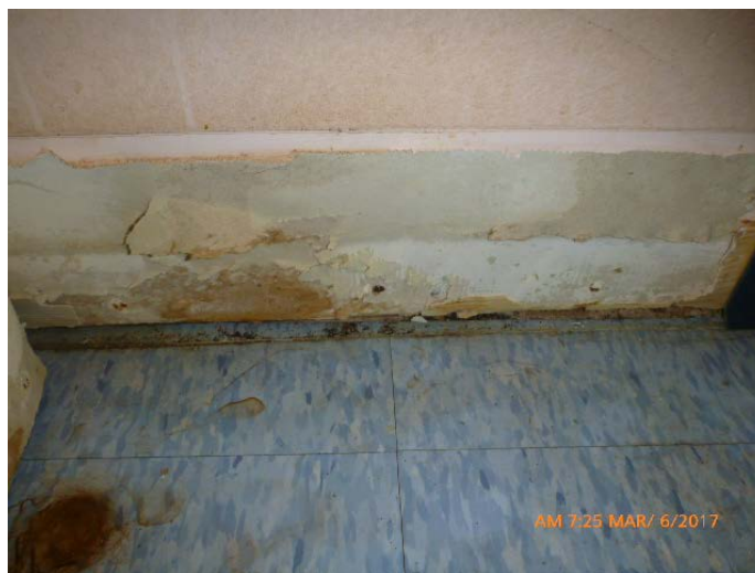
Photo #8: Close-up of base of wall and moisture impact. Staining observed on vinyl floor tile
