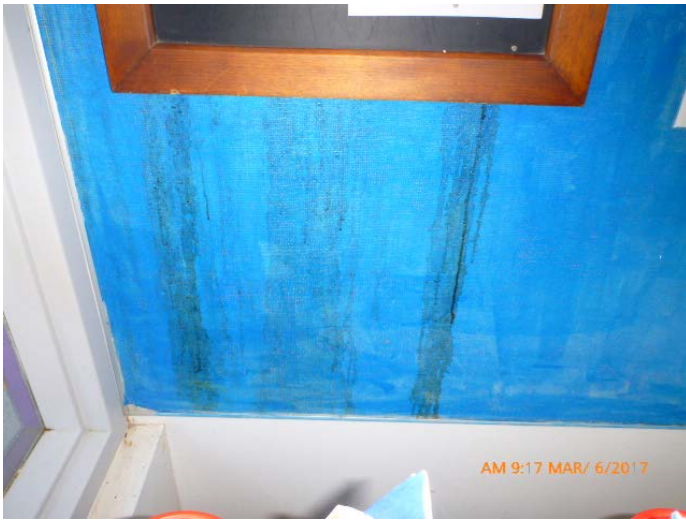
Photo 53: Staining observed approximately 3 ft' up along west wall outside bathroom
