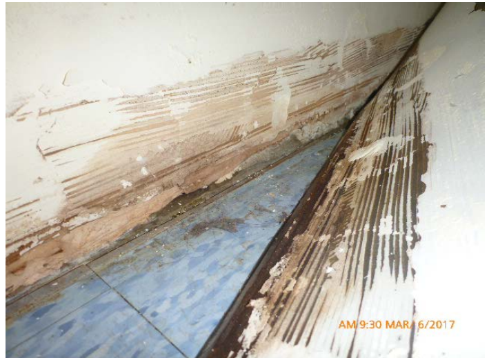
Photo 60: Moisture impact and mold growth observed along base of south and west walls
