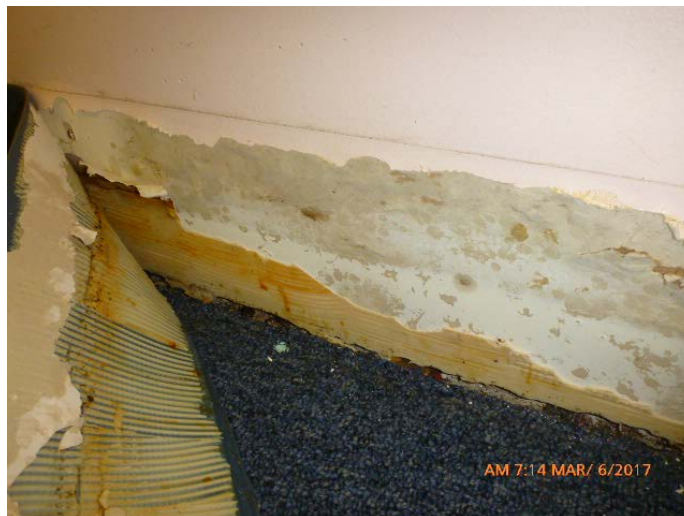
Photo #6: Close-up of base of north wall and moisture impact
