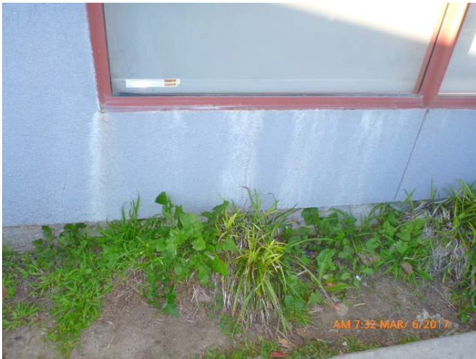
Photo #17: Staining observed below window along north perimeter
