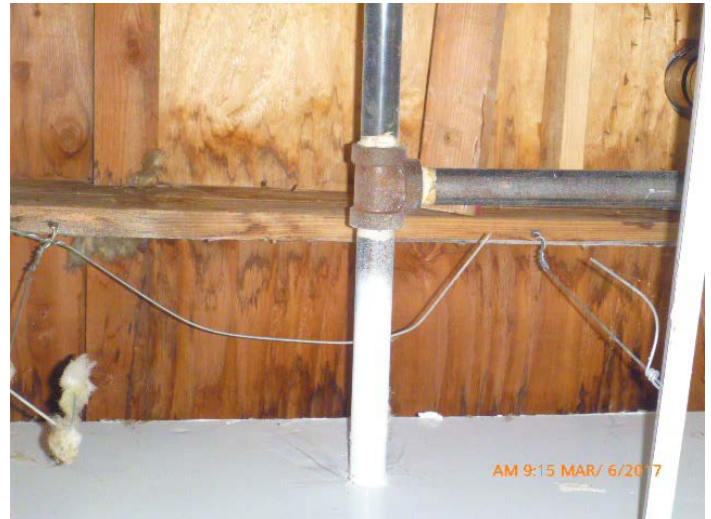
Photo 52: Roof drain and staining observed on exposed roofing materials
