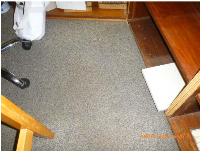
Photo 43: Stained carpeting observed along south perimeter
