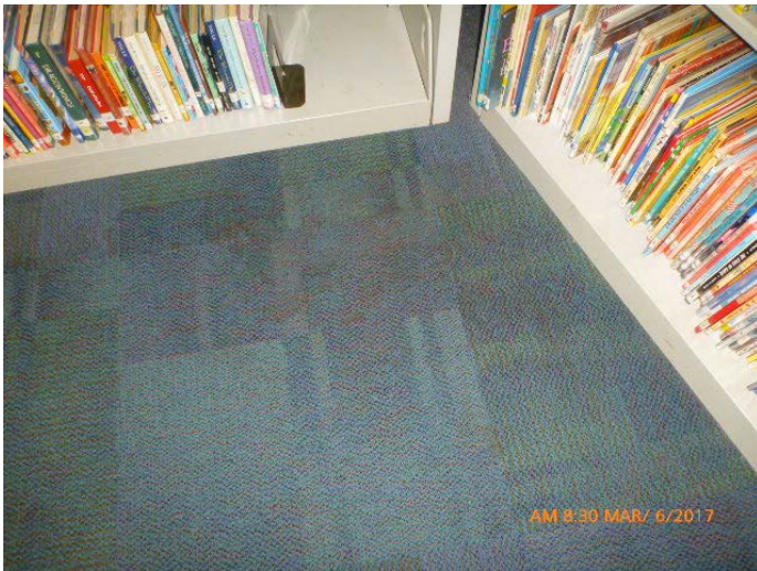
Photo #29: Overview of stained carpet in NW corner
