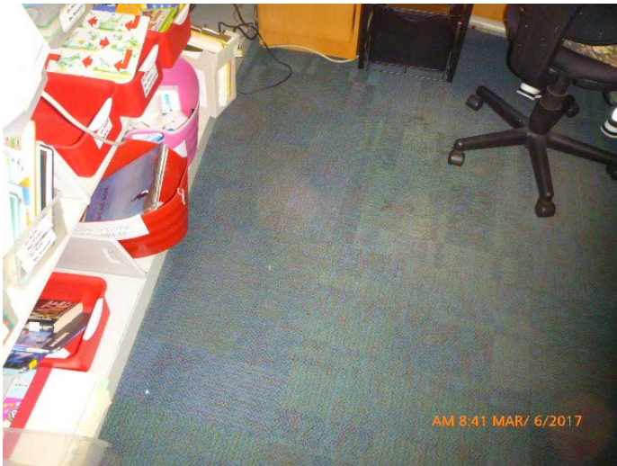
Photo #33: Stained carpeting observed along north perimeter
