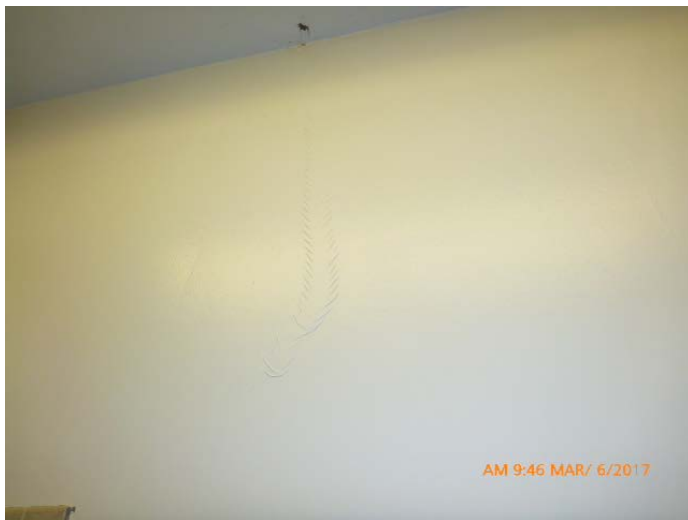
Photo 61: Moisture impact (e.g. bubbling paint) observed along west wall in bathroom
