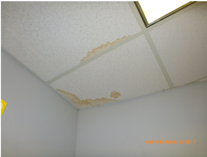
Photo 35: Stained ceiling tiles observed in SW corner
