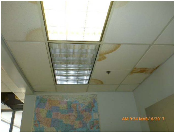
Photo 57: Additional stained ceiling tiles in SW corner adj. bathroom
