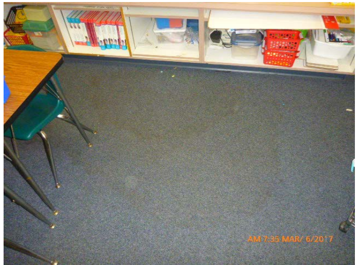
Photo #20: Stained carpeting along north perimeter
