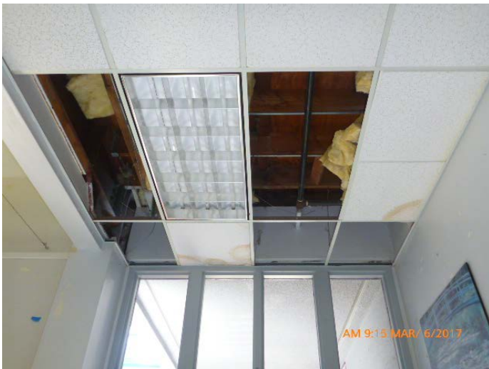
Photo 51: Missing and stained ceiling tiles observed in SW corner Adj. entry
