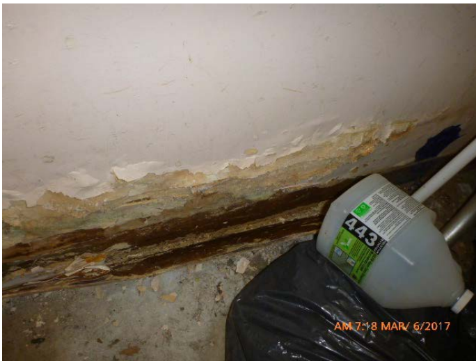
Photo #11: Heavy moisture damage, visible mold growth and elevated moisture along base of east wall
