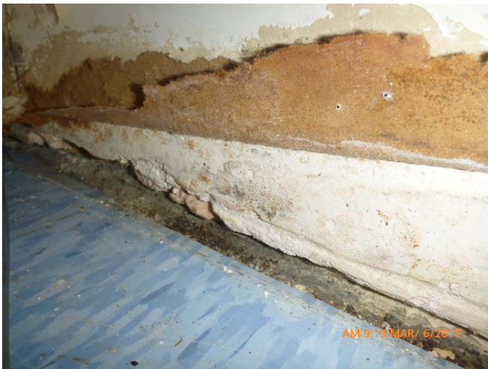
Photo 55: Mold growth and strong musty odors observed along base of west and south walls (both sides of ext. door)
