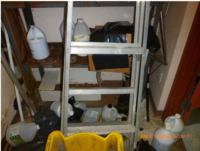
Photo #13: Additional moisture impact observed along base of south wall
