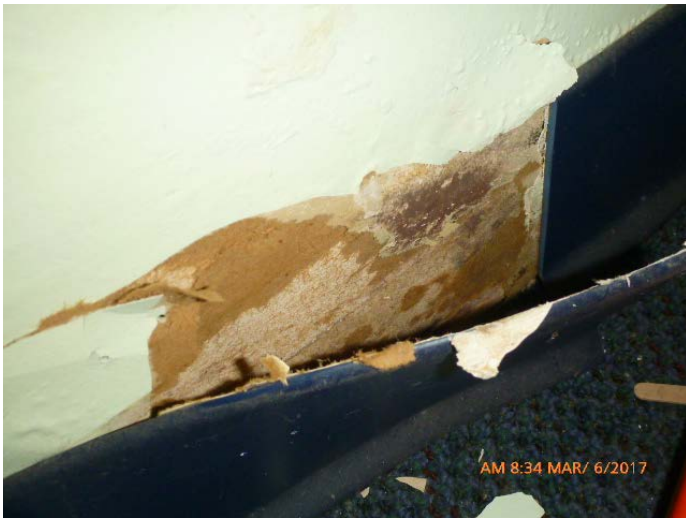
Photo #31: Mold growth observed behind base-cover on west wall
