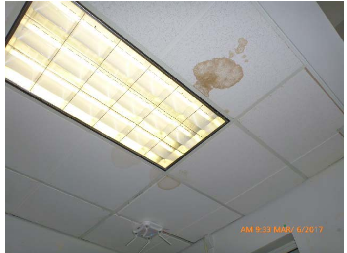
Photo 56: Stained ceiling tiles observed along north perimeter
