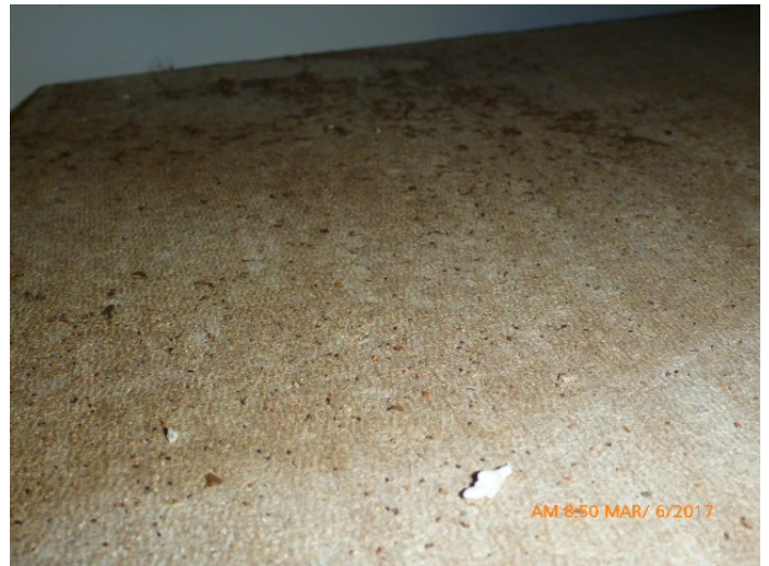
Photo 36: Overview of top of ceiling tile and staining/debris
